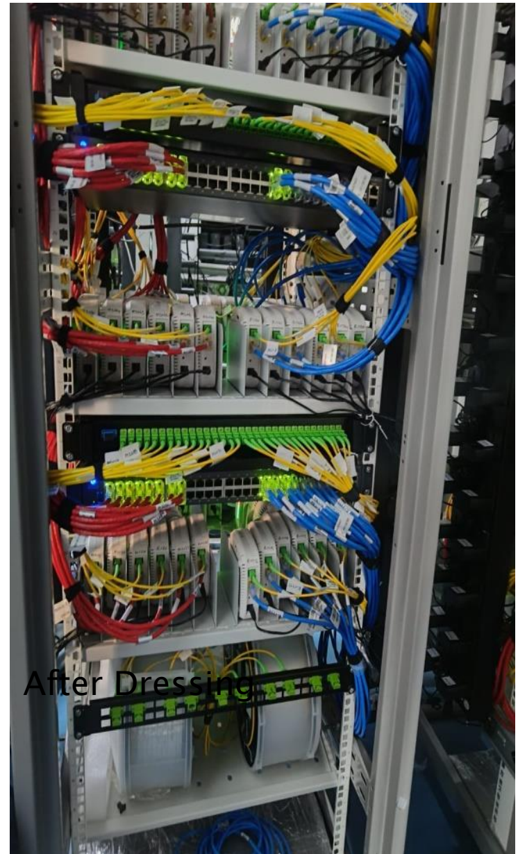
Structured Cabling Solution
